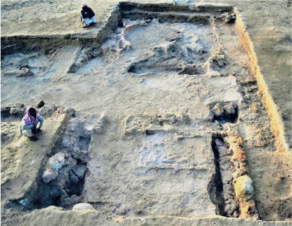
9. The western part of the bath with remains of Western Tholos ; view to the south (Phot. S.E. Sidebotham).
