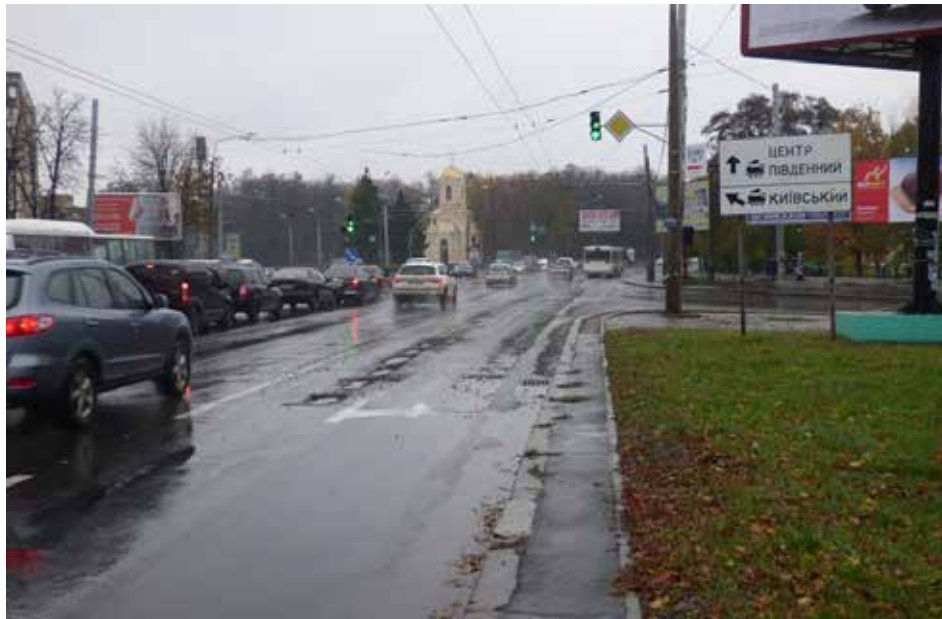
Figure 2. Damage to the road surface in Shevchenkivskiy district of Poltava
