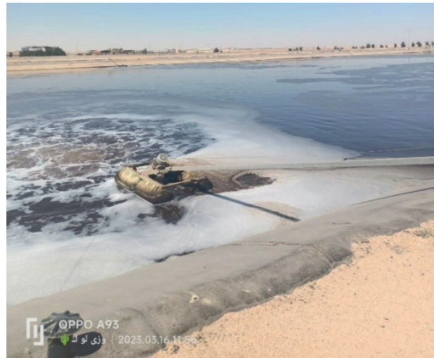
Fig. 7. Pump used by operators to absorb wastewater from the ground at the Oued Souf Wastewater Treatment Plant Source: Field internship for M1 students. Rural 2023
