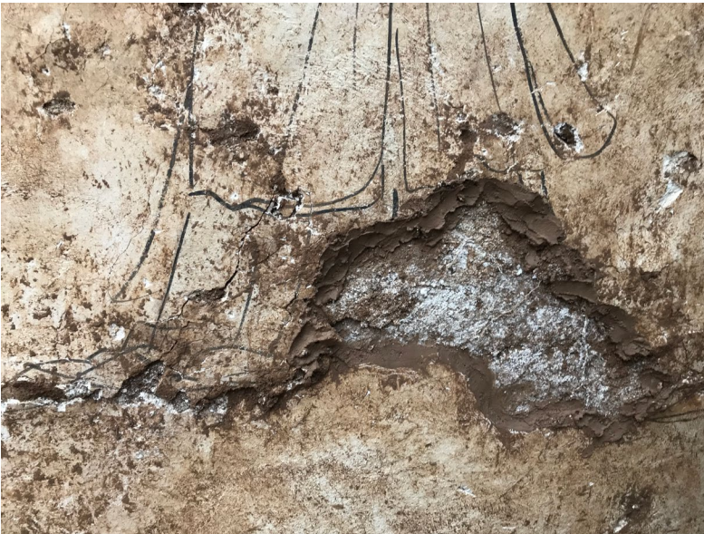
Fig. 9. The team was using the mud to spread on the breakage for reinforcement. Source: Author
