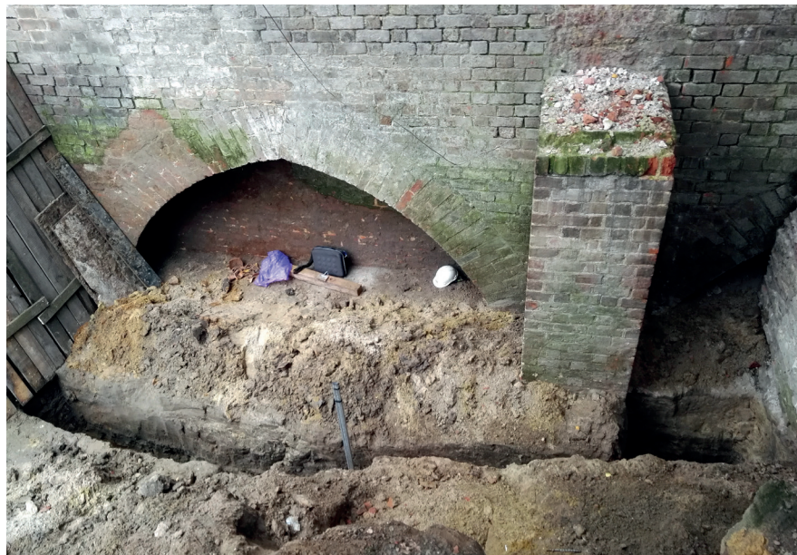
Fig. 8. Wrocław. The north end and the beginning of the middle span of the bridge seen together with the buttress. On the right side, the arched wall protected from mechanical damage (photo by P. Kmiecik)
