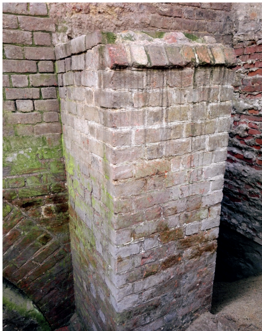
Fig. 10. Wrocław. The buttress: upper offset and arch connection are visible (photo by P. Kmiecik)
