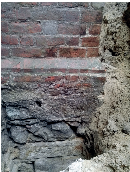
Fig. 11. Wrocław. Lower part of the buttress. Visible foundation technology and profiled offset made of brick fittings (photo by P. Kmiecik)
